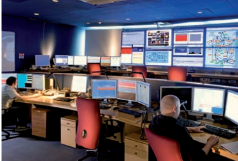
Network Operation Centres
